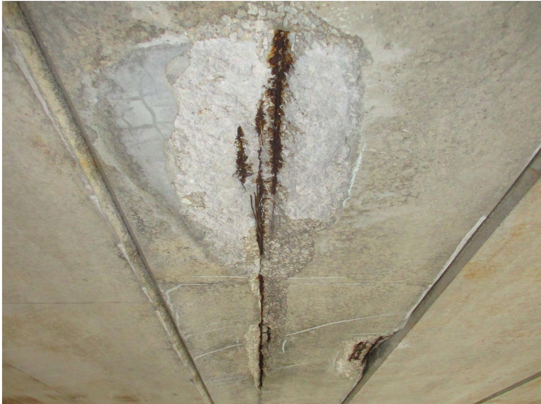
PPC beam spall with exposed and broken strands
