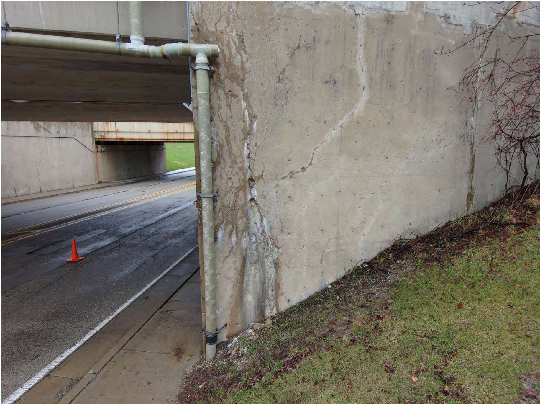
Southwest Wingwall map cracking and spalling
