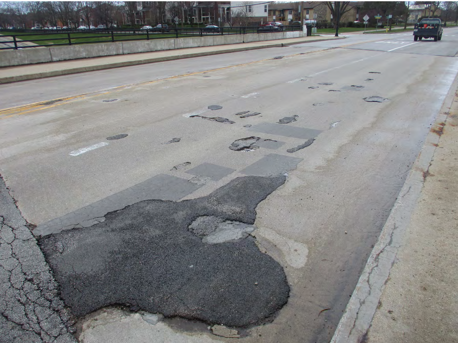
Typical deck condition with spalls with exposed reinforcement
