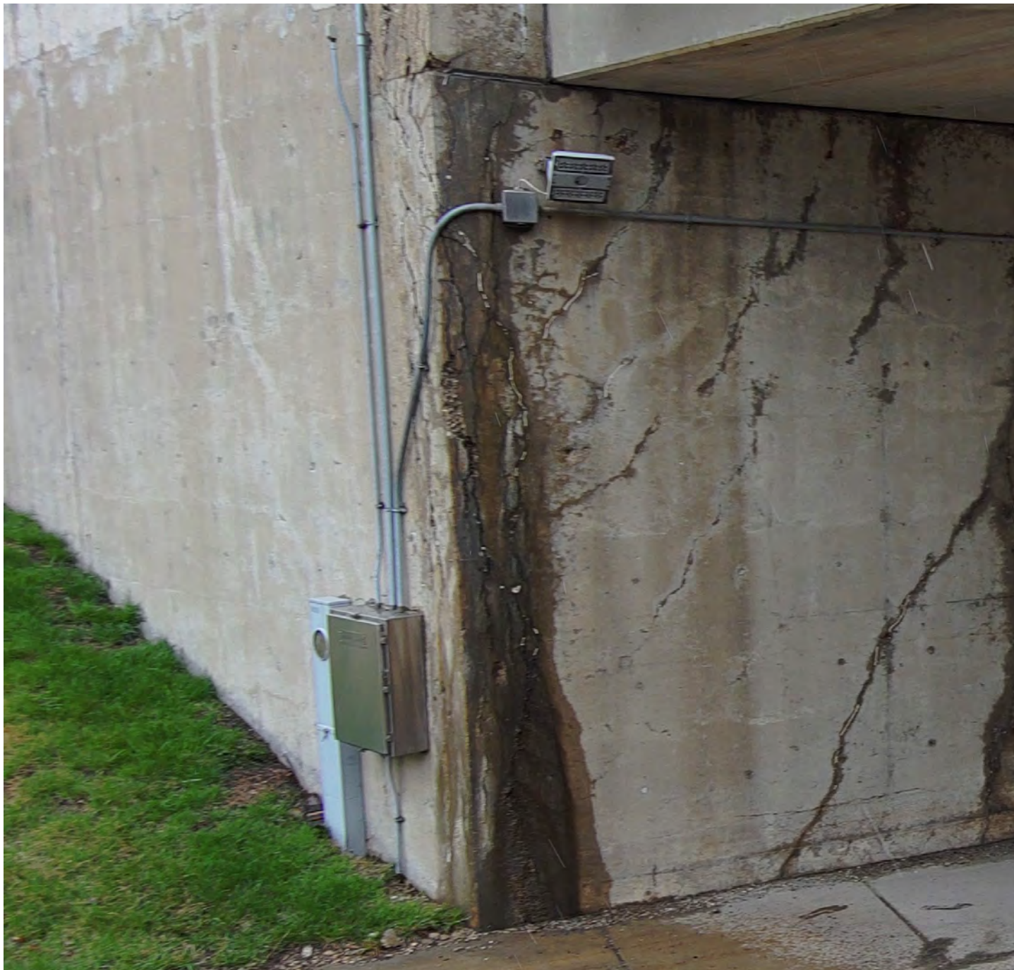
Northwest Wingwall map cracking, delaminations, and spalling
